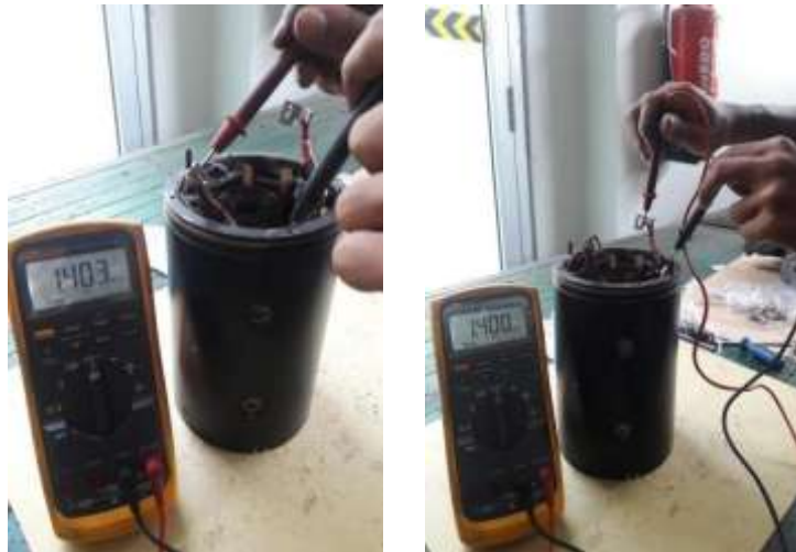
Gambar 9. Pengujian Field Winding Ground
