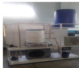
Gambar 4. Sistem instalasi Air Conditioning Water Heater (ACWH): 1. Tangki pengisi; 2. Tangki pemanas air (APK); 3. Condensing unit ; 4. Pompa air; 5. Power panel
